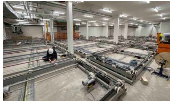
Automated Parking Installation
